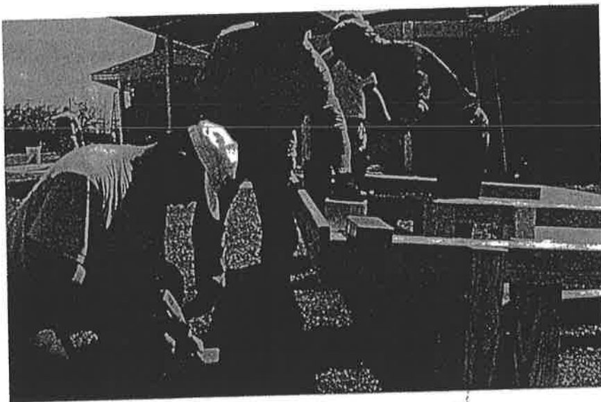
During a Presbyterian Men service day in Detroit, volunteers do construction work at Park United Presbyterian Church.
